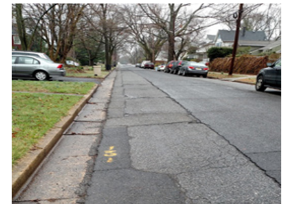
Surface Defects and Cracking
