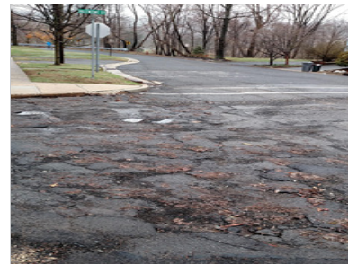
Potholes & Deteriorating Patching
