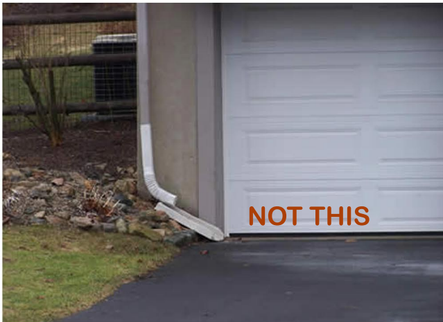
Downspout directs rain to the driveway and street; rain becomes stormwater runoff.
