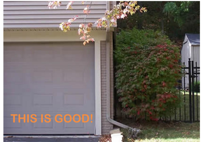
Downspout directs rain to landscaped area; rain soaks into the ground.
